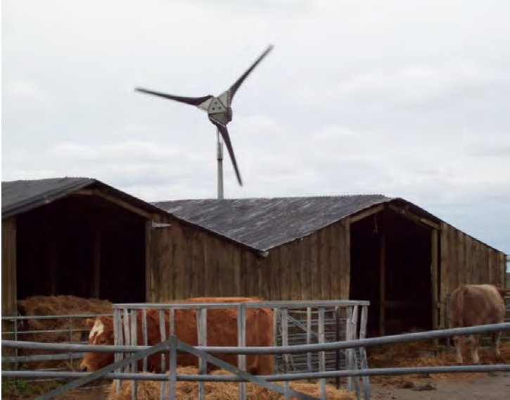
6kW wind turbine
