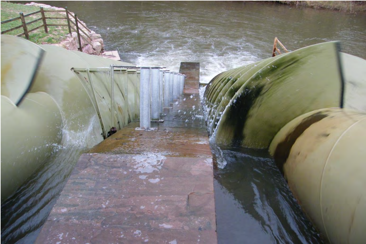
Osbaston Hydro project, Monmouthshire – Archimedes screw system Image source: Monmouthshire County Council
